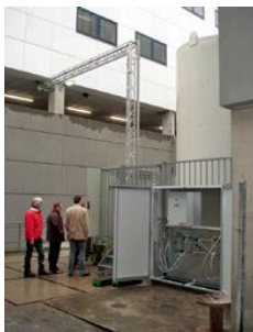
Filling station CryoMat
