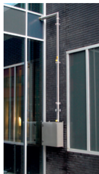
Filling box on the ground floor
